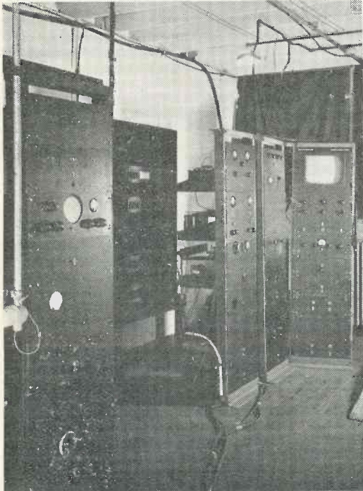
The racks containing the scan generators line amplifiers, synchronising generators and monitor tubes.
