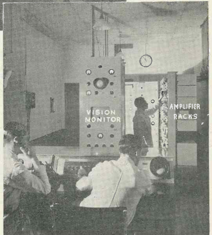
Baird Control Room. Centre background: Vision monitoring panel. Right: Amplifier racks. Foreground: Control desk.
